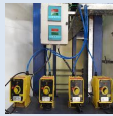
pH dosing system
