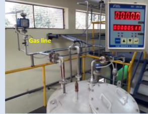
Gas collection & online monitoring system
